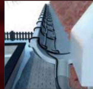
Trace Gutter Heating Cables (SNOW/ICE MELTING)
